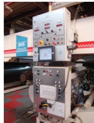
Rollstand operator touch screen.
